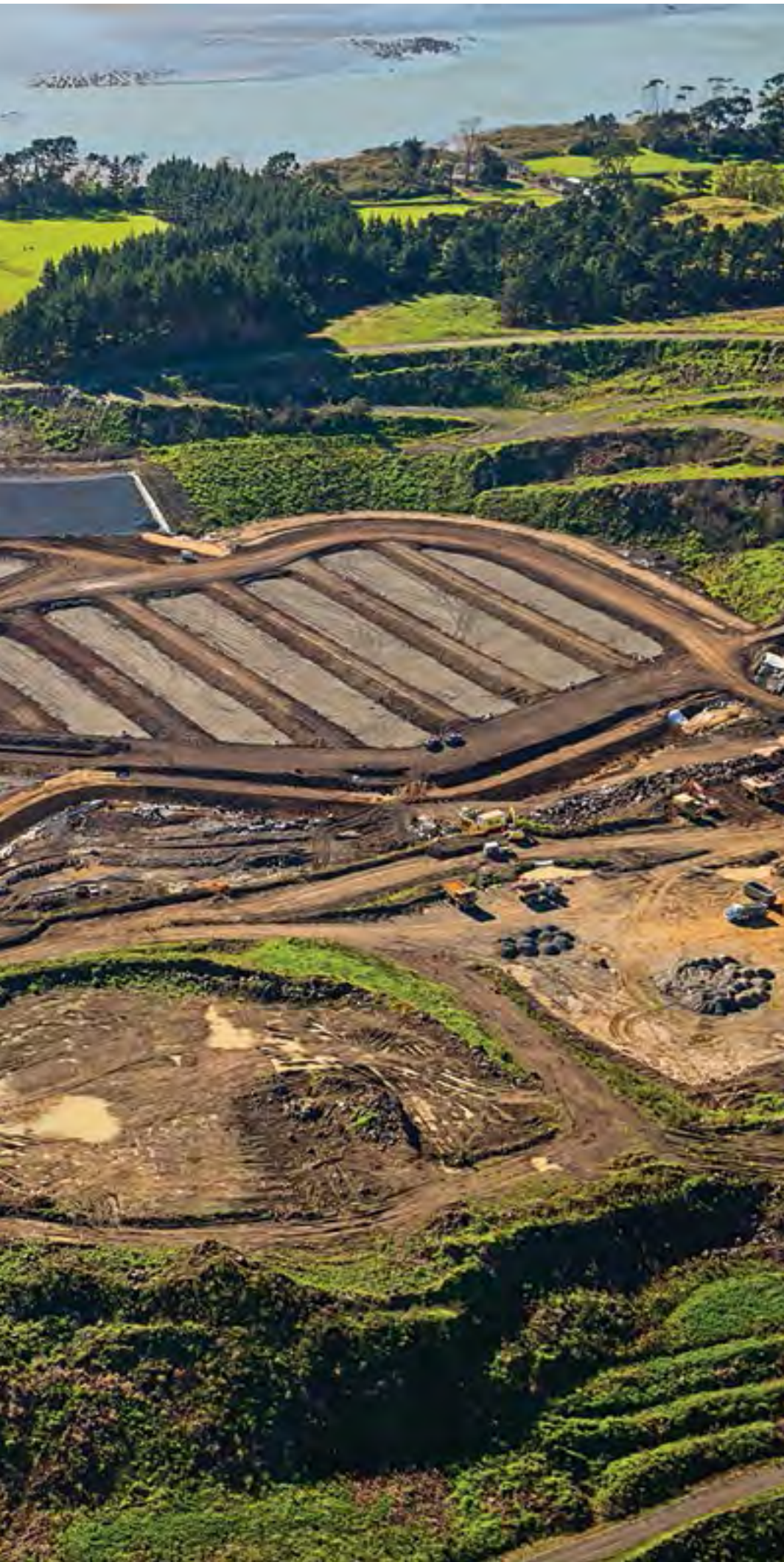
Aerial view of Puketutu Island, where Phase 1 of capital works has been completed and the facility is ready for placement of biosolids from Mangere Wastewater Treatment Plant.
